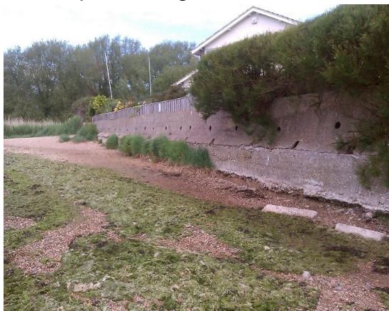
Plate 3: Seawall undercutting area
