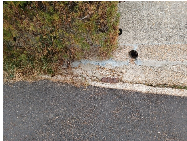
Plate 7: vegetation and drainage holes over seawall
