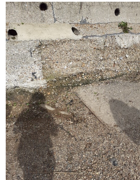
Plate 11: spalling of face and undermining of wall
