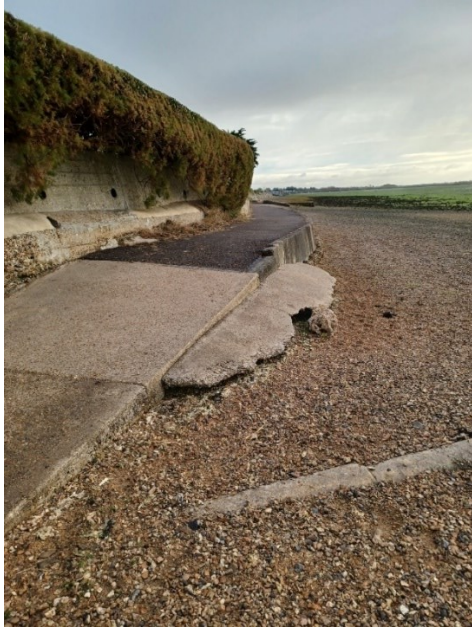
Plate 9: undermining of concrete slab on footpath
