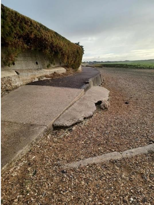
Plate 9: Beach lowering undermining ramp toe protection
